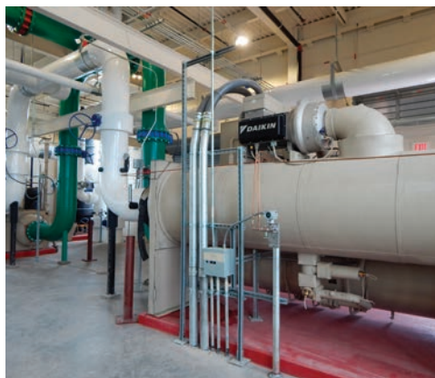
High efficiency magnetic bearing chillers in Terminal Airside 4 at Orlando International Airport.
